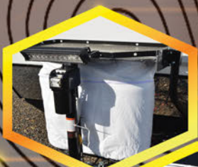
10 Gallon LP Tanks
